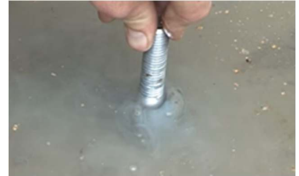
Wet and Water-Filled Holes
